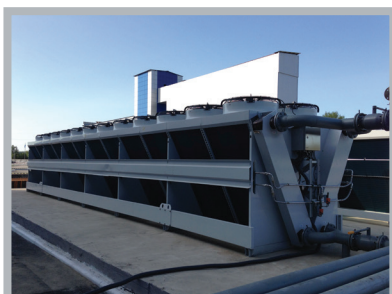
free cooling chillers
