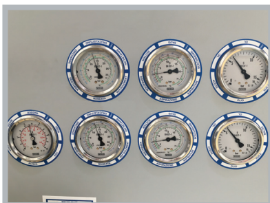
refrigerant and oil gauges
