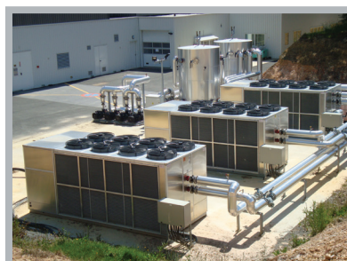
high capacity process chillers
